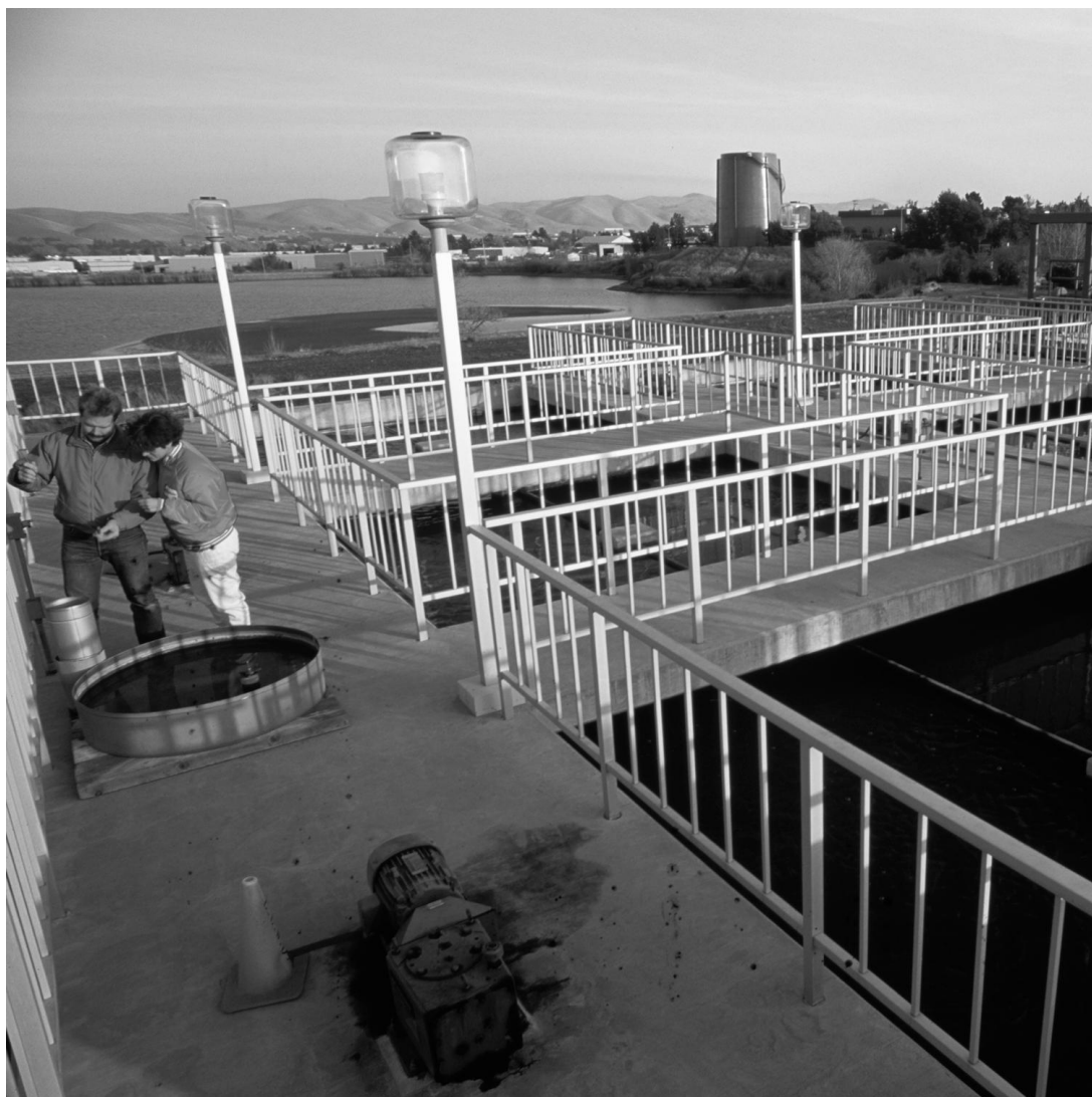
A WATER FILTRATION PLANT IN CONTRA COSTA COUNTY, CALIFORNIA. (James A. Sugar/Corbis. Reproduced by permission.)
